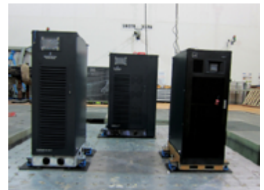
Dynamic/functional tests on UPS systems
