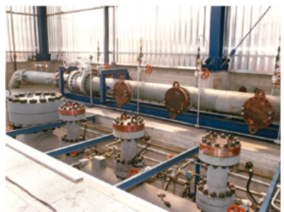
10" and 24" flanges for the installation of valves to be tested
