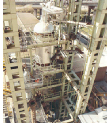
GEST plant vessel (volume 43 m 3 , height 15 m)
