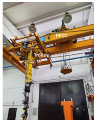
DRP hall – Carro ponte, trolley e PFCT
