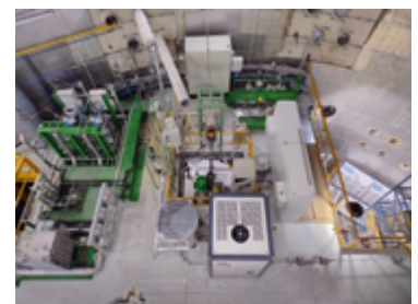
CIRCE facility (top view): auxiliary systems and components
