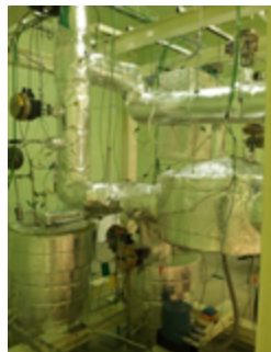
View of the Lifus 6 facility
