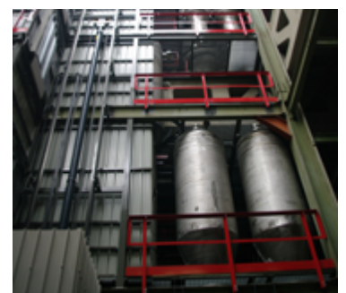
SPES-3 experimental facility: view of containment compartment tanks (total height 30 m)
