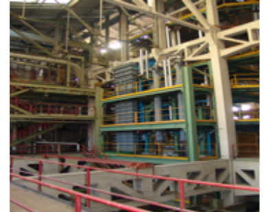
SPES-2 experimental facility: view of passive safety systems (total height 30 m)
