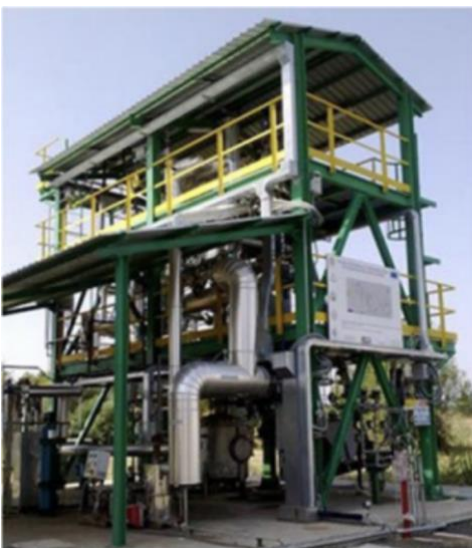
Figure 5 - The updraft fixed bed gasification plant
