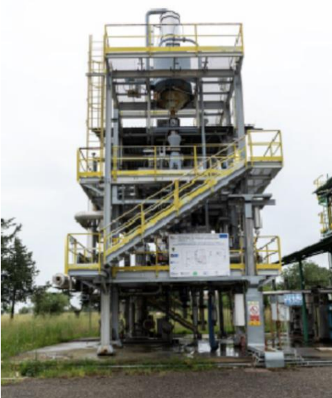
Dual fluidized bed gasifier - Steam 500kWth
