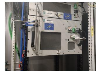
Figure 2 Installed electrolyser at ZEM module
