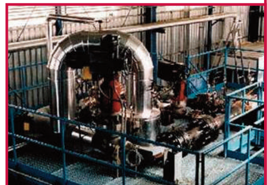
Test of the automatic Depressurization System of the AP-600 reactor (Westinghouse). Overall view during a phase of the experimental campaign
