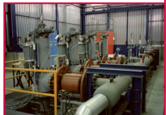
Set of 4 Safety Relief Valves (to be installed on the former "Montalto di Castro" NPP, Italy) mounted for testing on the VAPORE plant
