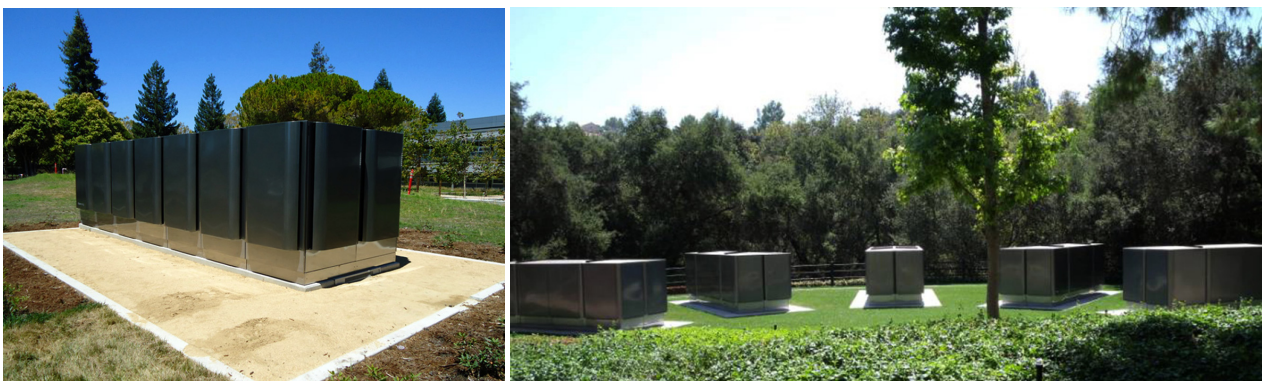
Figure 15. Bloom Energy Servers at NASA and the Federal Bank of America. [source: Bloom Energy, www.bloomenergy.com ]
