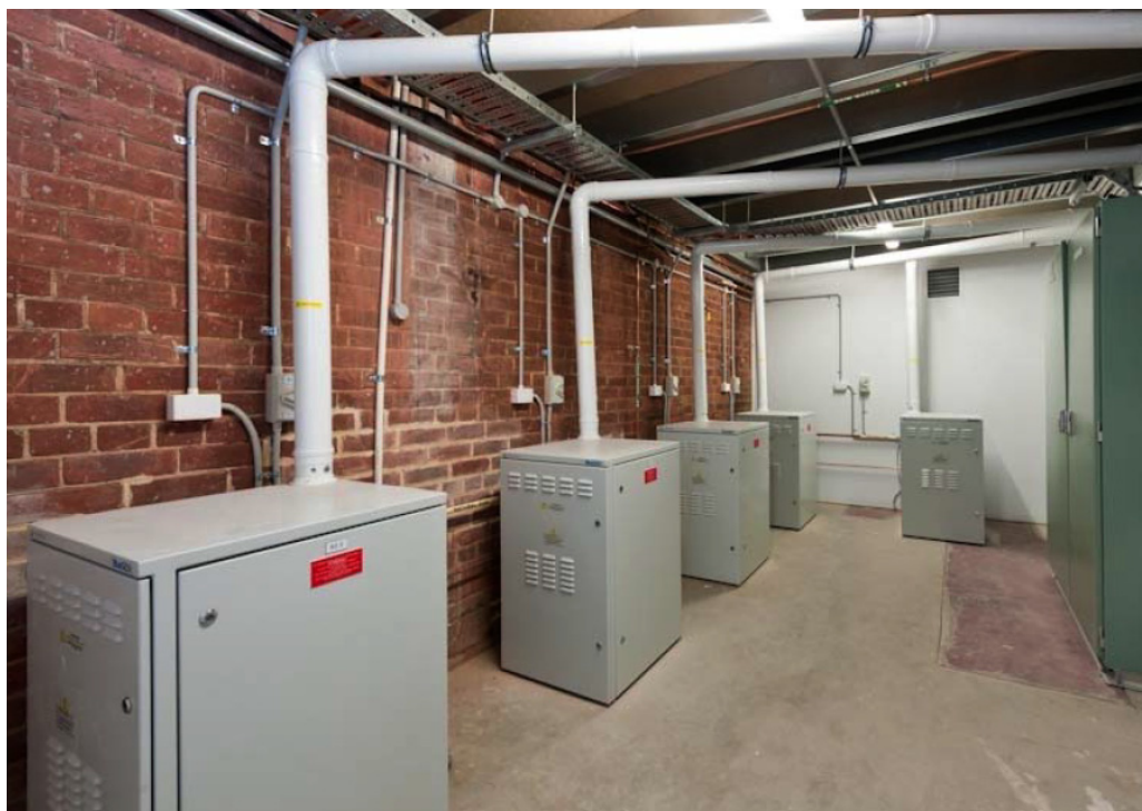
Figure 46. BlueGens installed in March 2012 as retrofit of a Commercial building in Adelaide (over 7 tonnes of carbon saved in first 3 months). [source: CFCL, Clean Power for Global Markets Shareholder Update 2012]
