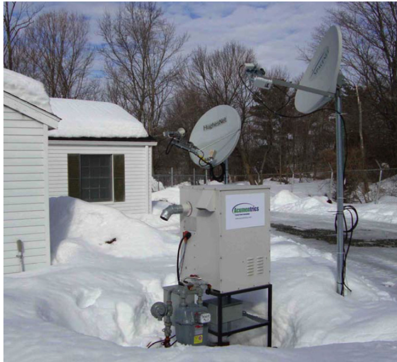
Figure 12. An example of remote, stand-alone power supply.
