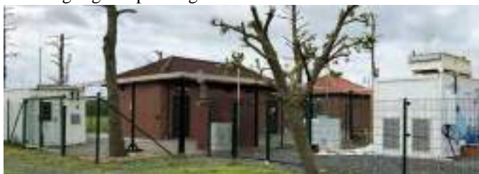
Fig. 1. HPEM2GAS Water electrolysis plant installed in Emden (Germany)
