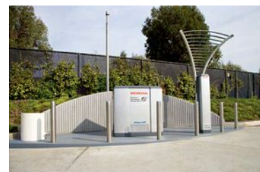
Home Energy Station IV - Honda / Plug Power (Torrance, CA, USA)
