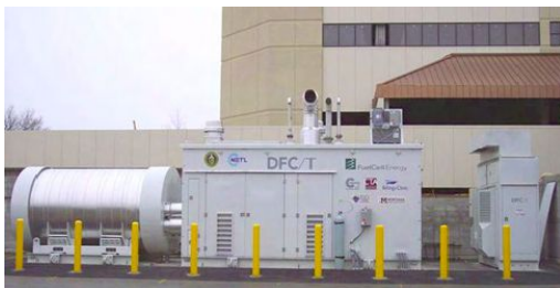
Impianto DFC/T®, Billings Clinic (MT, USA)
