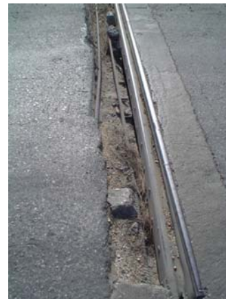
Figure 4. Damage at a joint on the bridge deck.
