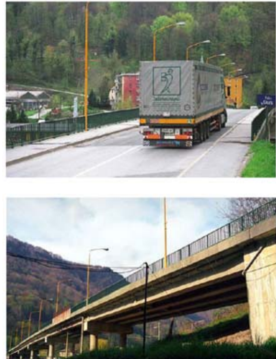
Figure 1. Site of the SAMARIS (2006) study, the Hrastnik Bridge in Slovenia. Top: View of the bridge from above. Bottom: Side view of the bridge. Source: SAMARIS (2006).
