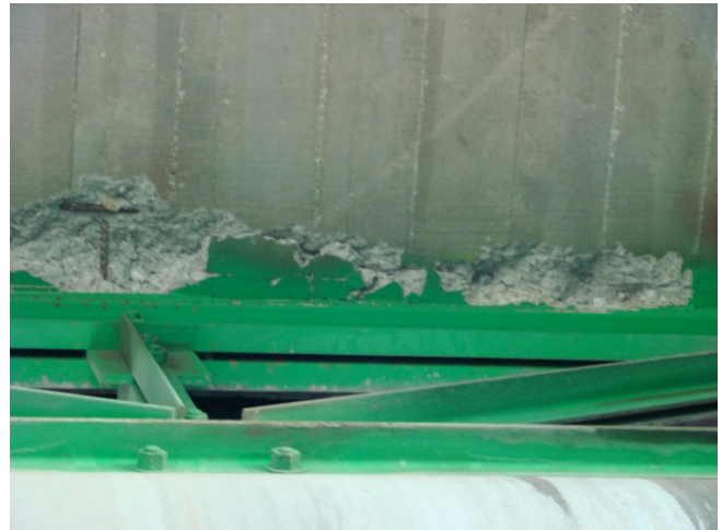
Figure 3. Scarps under the deck near a joint, due to stress concentration.
