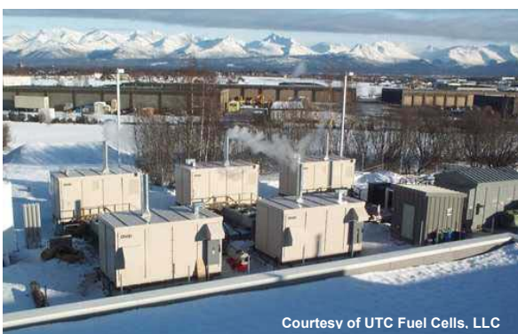
1 MW Fuel Cell Project, US Post Office, Anchorage, Alaska
