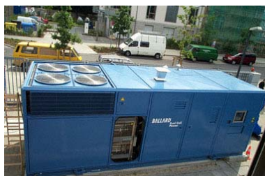
Impianto Ballard 250 kW, Bewag Treptow Heating Plant, Berlino
