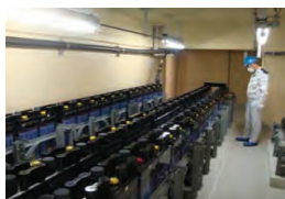
125V battery charger room
