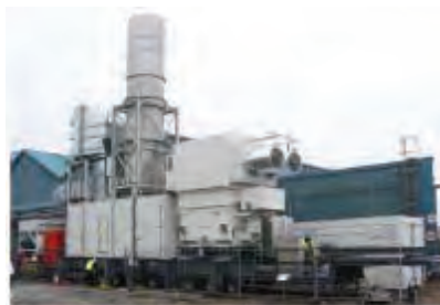
Gas turbine generator (Source: The Chugoku Electric Power Co.,Inc.)
