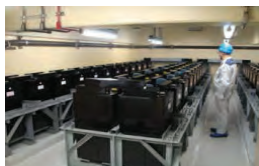
250V battery charger room
