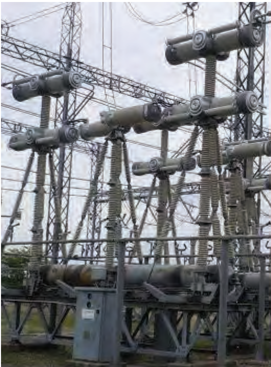
275kV air blast breaker (ABB) (Source: Electrical Equipment Earthquake Countermeasures WG)
