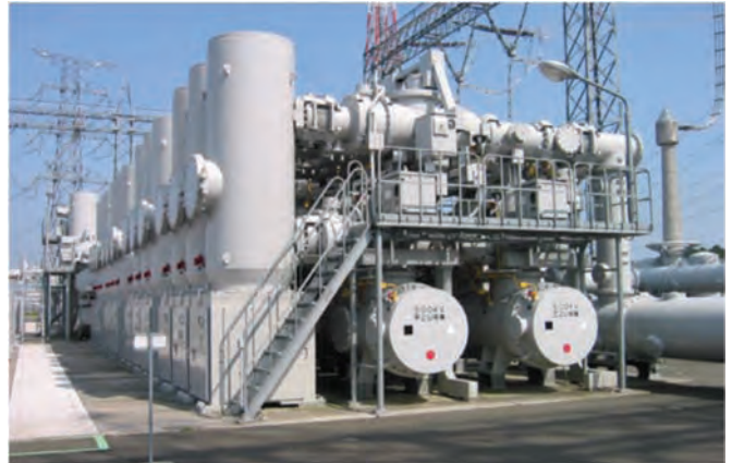
550kV gas insulated switchgear (GIS) (Source: Japan AE Power Systems Co. website)
