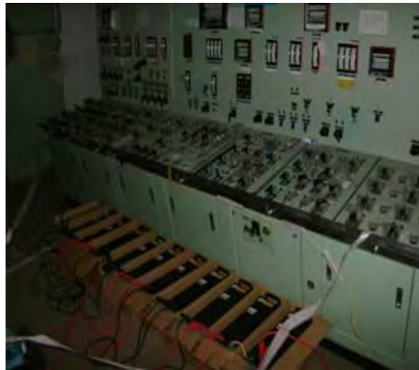
Figure 3 - Batteries connected to instruments in the MCR
