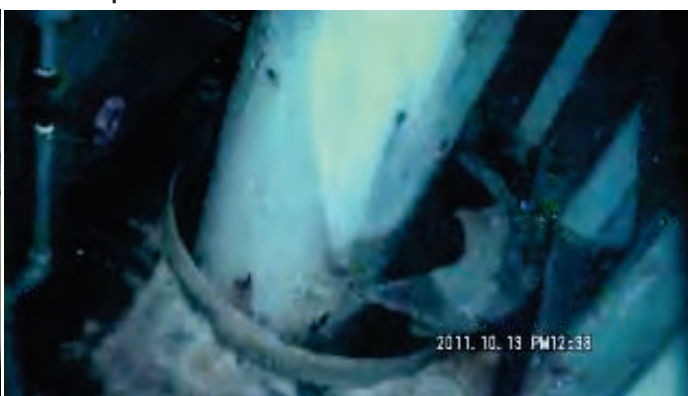
Situation of the penetration on 1 st floor with no steam release (photo as at Oct. 13)
