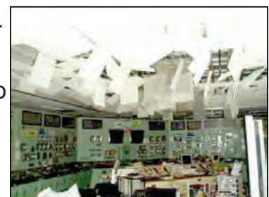
Unit 1 Main Control Room
