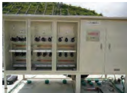
Power supply inlets outside of the buildings (Source: The Shikoku Electric Power Co.,Inc.)
