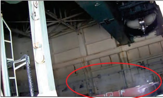
Steam release from right above the reactor on 5 th floor (photo as of Sep. 17)
