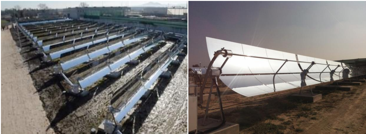
Figure 3 – Photo of the solar thermal plant and detail of a parabolic trough (right)
