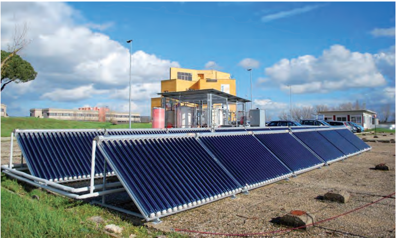
Solar cooling and heating in the Casaccia test building
